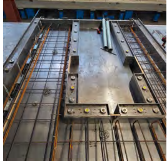
SAS recess solution – shutterings placed by the robot are manually supplemented with custom-made plywood
